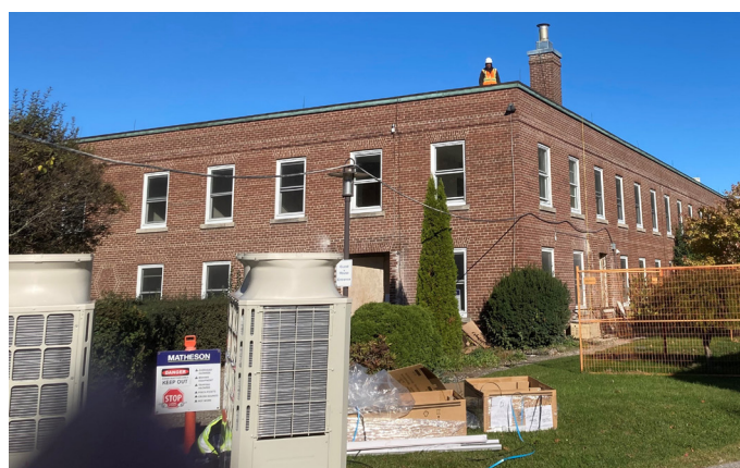
HVAC units ready to be installed
