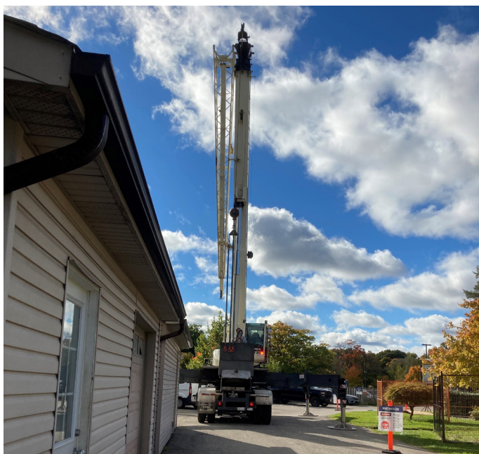
Crane and HVAC systems
